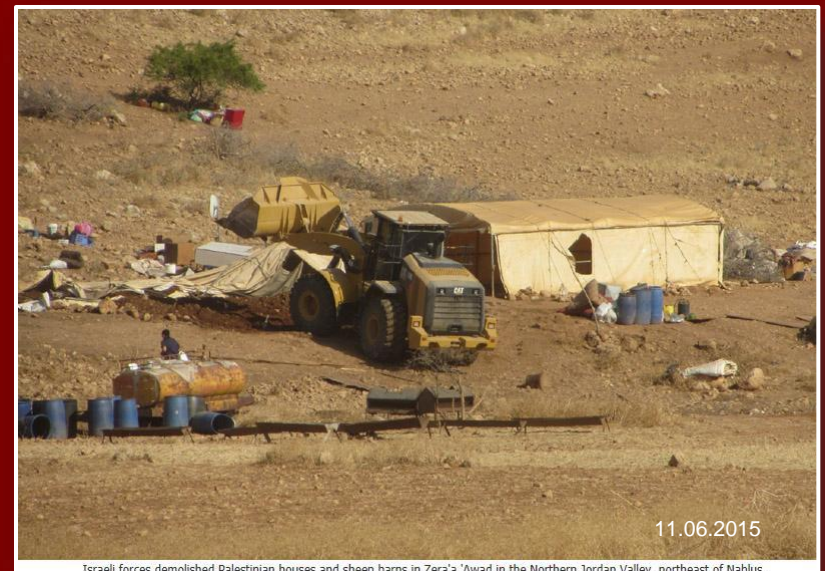
Israeli forces demolished Palestinian houses and sheep barns in Zera'a 'Awad in the Northern Jordan Valley, northeast of Nablus.
