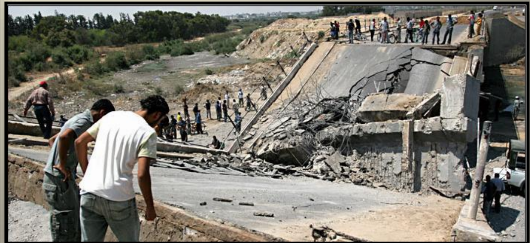
Bridge destroyed in Gaza, 28.06.06
