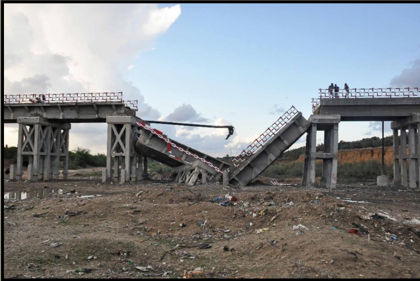
A pedestrian bridge destroyed by Israeli air strikes in the Al Mughraqa area of the Gaza Strip
