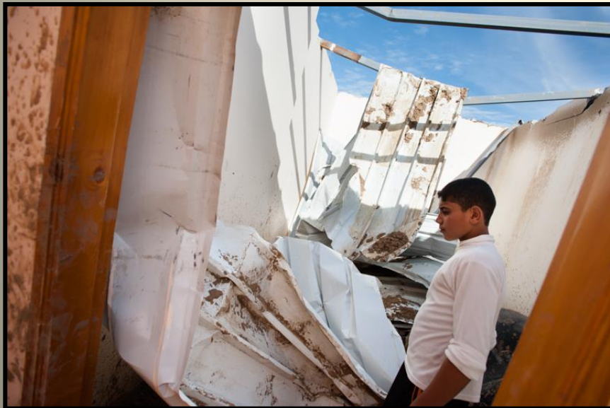
The roof of this house was destroyed by debris thrown into the air by Israeli bombings in the Al Shoja'iya area of Gaza City.
