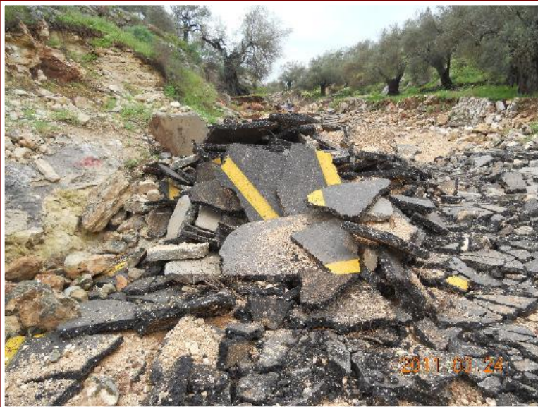
This 2 km long Palestinian road, was destroyed in Qarawat Bani Hassan on 23 March 2011.
