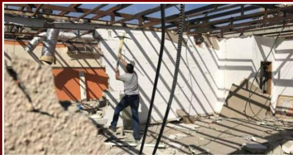
Dalia Julani family are forced to demolish their own house, in the Arab town of 'Ara, Haifa District, September 2019
