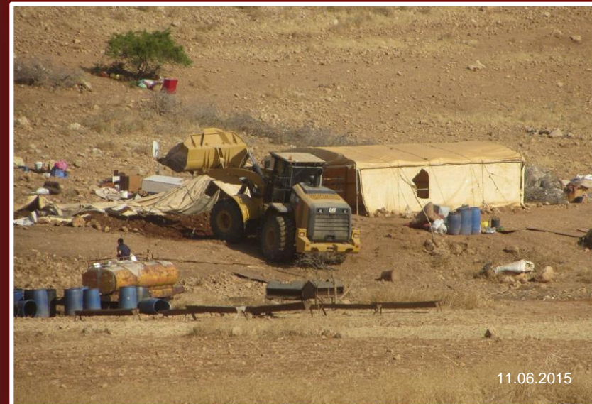
Israeli forces demolished Palestinian houses and sheep barns in Zera'a 'Awad in the Northern Jordan Valley, northeast of Nablus.
