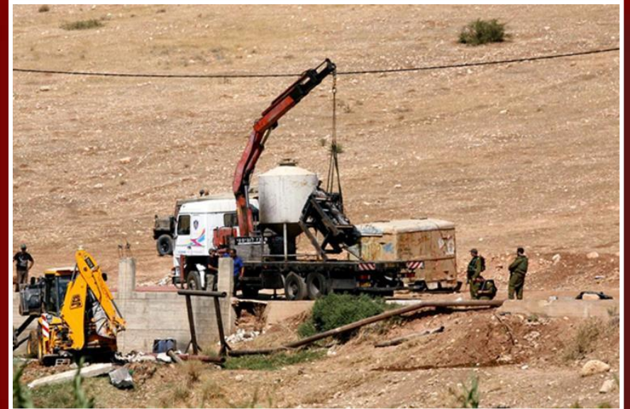
Demolition of a water well and equipment confiscation in An Nasariya, Jordan Valley. September 8, 2011
