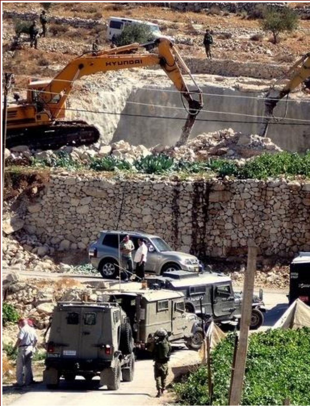
Demolition of a palestinian water- reservoir in al Baqa North of Hebron, 03.09.2009
