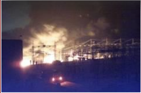
The power plant of Baslim in Lebanon destroyed by the israelis in may 2000
