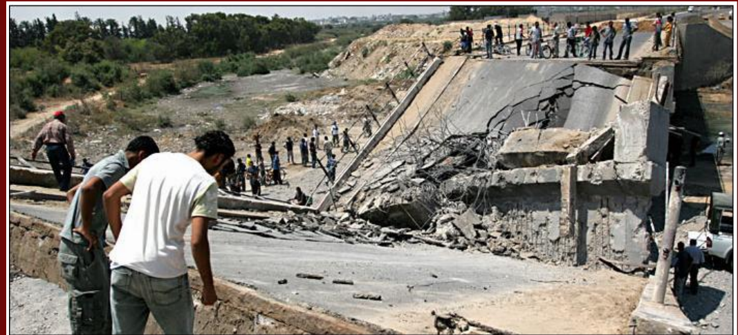
Bridge destroyed in Gaza, 28.06.06
