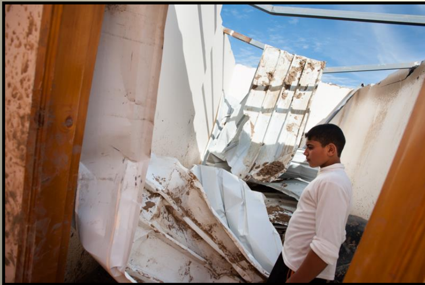
The roof of this house was destroyed by debris thrown into the air by Israeli bombings in the Al Shoja'iya area of Gaza City.
